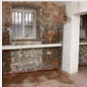
On damp masonry
