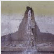
For water bearing cracks
