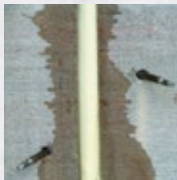
Forms foam in wet cracks
