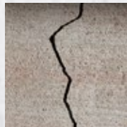
For dry cracks
